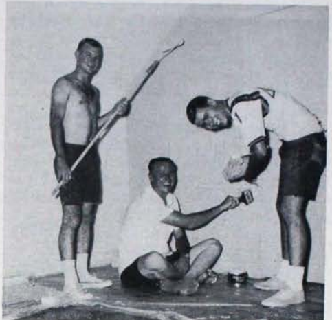
THE BETA UPSILON CHAPTER Lodge at Texas Tech receives a new coat of paint from Brothers Jim Choate, Larry Schultz, and Charles Giddens.
