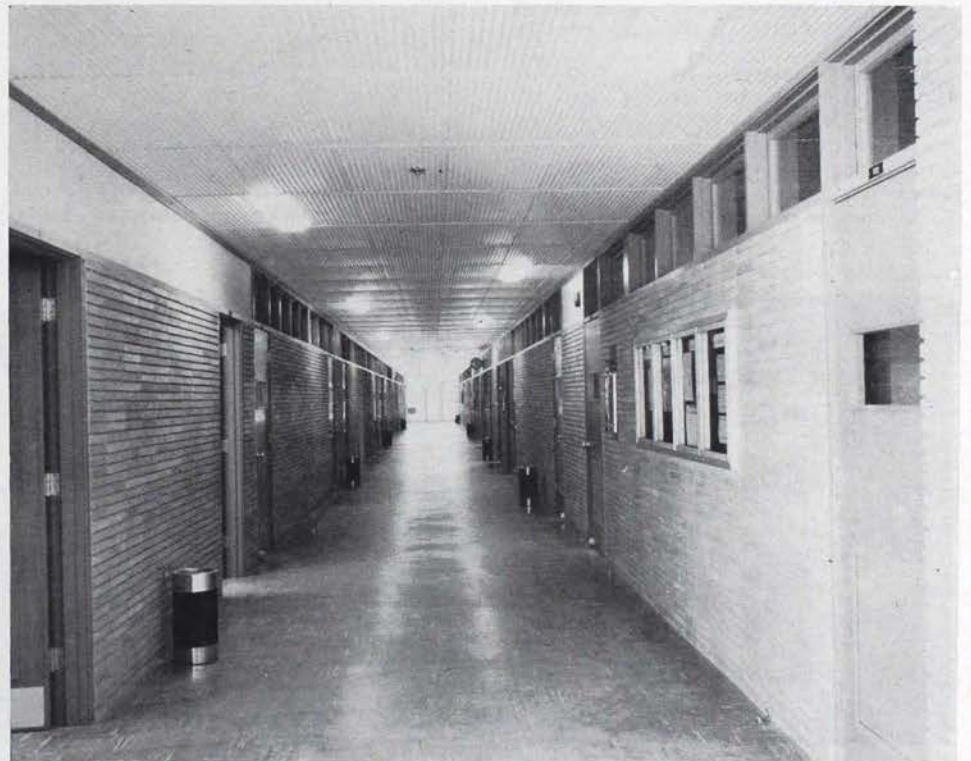
THIS SPOTLESS CORRIDOR keynotes the entire building of the School of Business at Lamar Tech.
