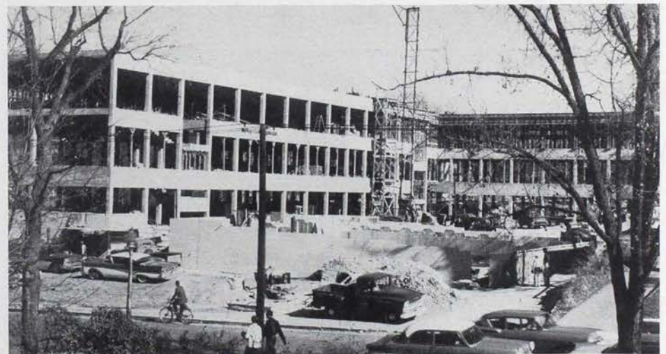
UNDER CONSTRUCTION is the new Business and Public Administration Building on the University of Missouri Campus. It is due for completion and use about September 1959.
