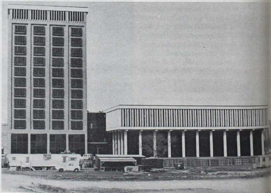
STILL SHOWING SIGNS of construction is the new home of the School of Business Administration at Texas Technological College in Lubbock, Texas. The building was recently completed at a cost of $4.5 million.
