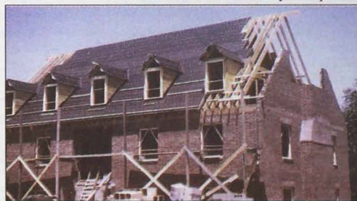
Construction began in November 1955 with a completion date of May 1956. A severe winter handicapped the builders for several months and the date was pushed back to September 1956.
