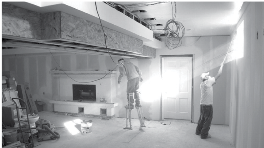
Previously unfinished, the basement will feature office space, beautiful new display cabinet, and an impressive board room.
