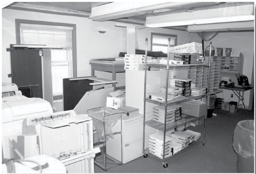
Extensive interior remodeling with an occupied building requires much "shifting about." The area above was cleared for asbestos remediation, then packed full of equipment, and on February 28 cleared out again.
